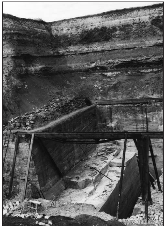
Figure 5. Thompson's Ancaster Stone Quarry, Wilsford Heath, Ancaster, with 4.5 m of Rutland Formation clays and sands overlying thickly bedded Ancaster Stone of the Lincolnshire Limestone (BGS photo #A6333, 1933).
